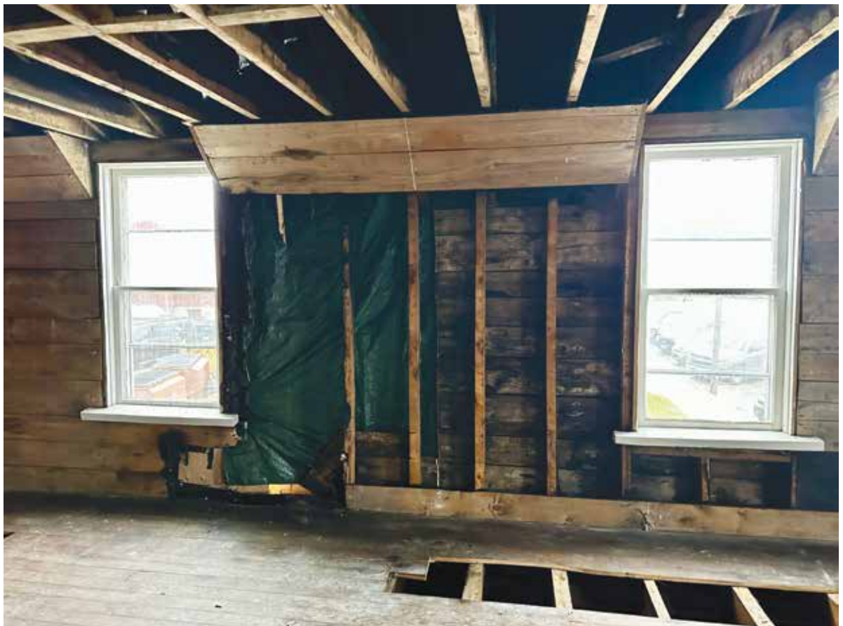
► On the second floor, the fire spread through the floor, wall and ceiling. PHOTO BY TONY AGUILAR.
